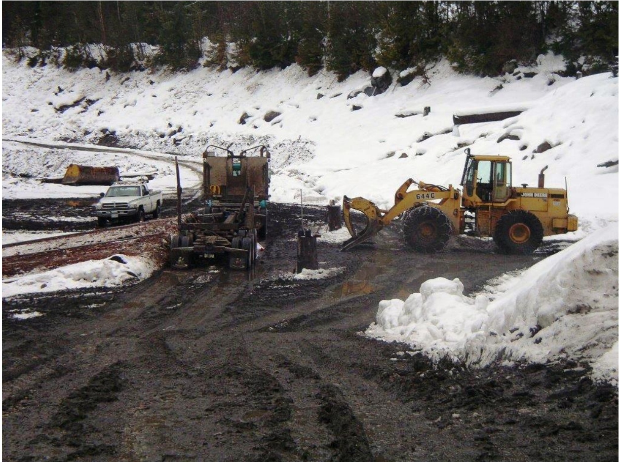
The above picture is an overview from the incident site
