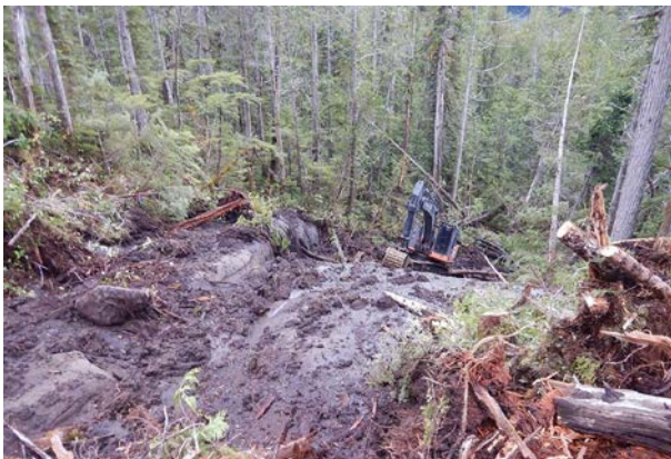
Excavator in a construction initiated slide.
